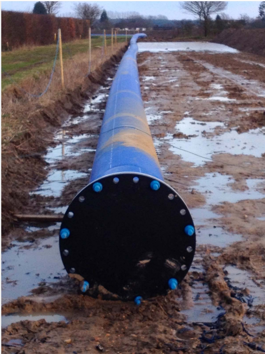
Crossing Boxted Public Footpath 38 the new water main being installed between Langham and Gt Horkesley by Anglian Water.
